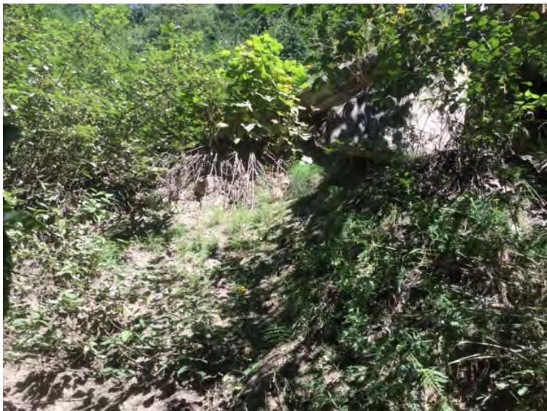
Downstream right fill slope eroding
