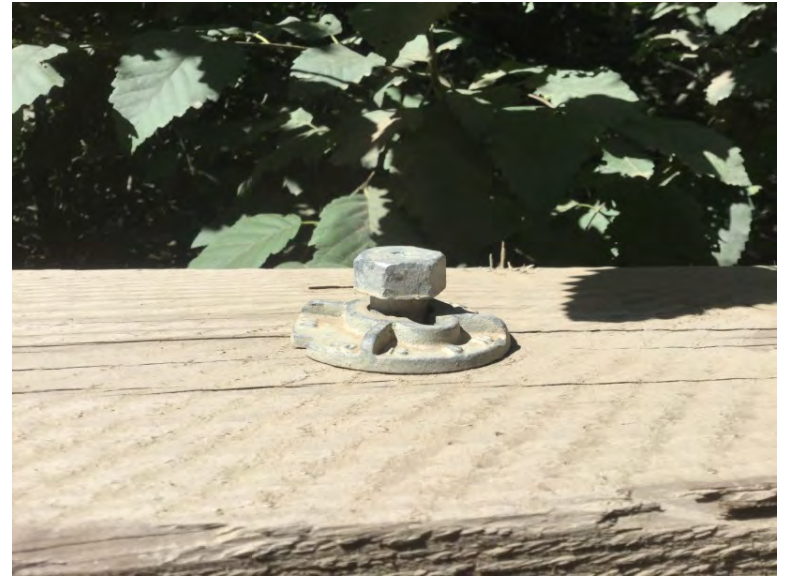
Loose rail bolts throughout
