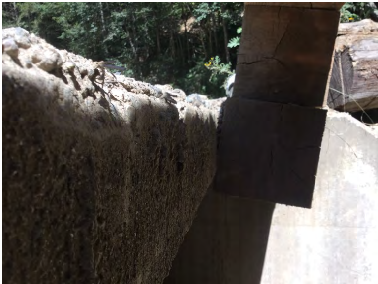
Upstream right bank blocks, risers and rail has been pushed out
